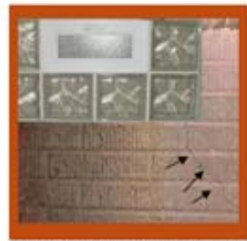
Typical Reentrant Crack
